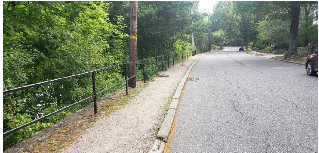
Improve curbs to improve street drainage and curtail bank erosion
